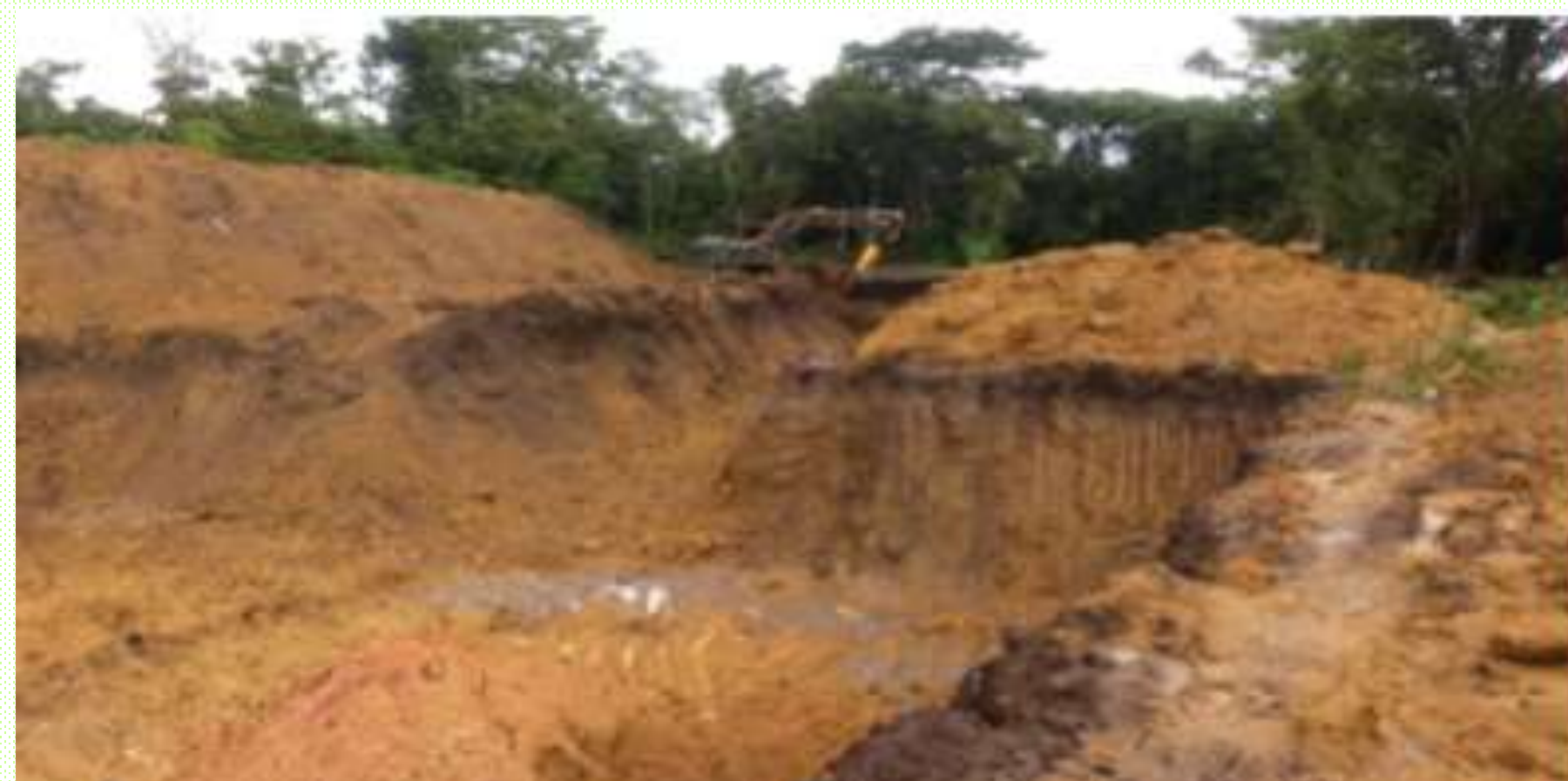
Image 2- Holes dug by hydraulic backhoes that dig the banks of the rivers in search of gold and destroy the riparian forests
